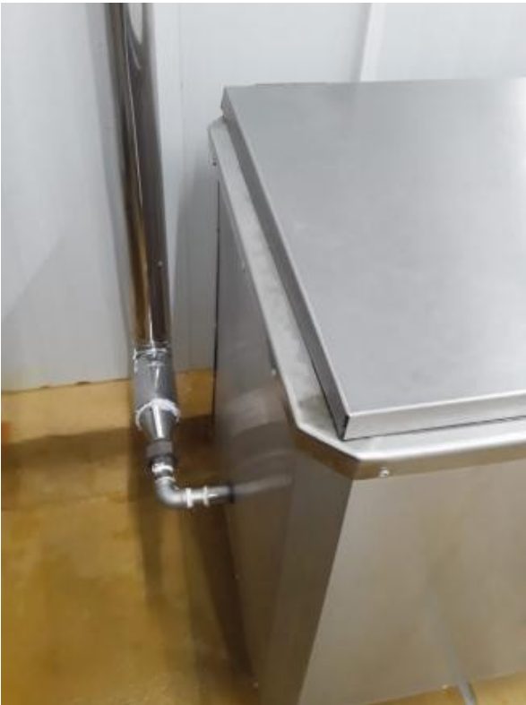
Stainless steel fabricated unit and pipe connection
