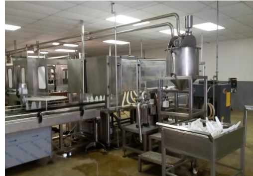
Packo Foods - Process equipment and pipework
