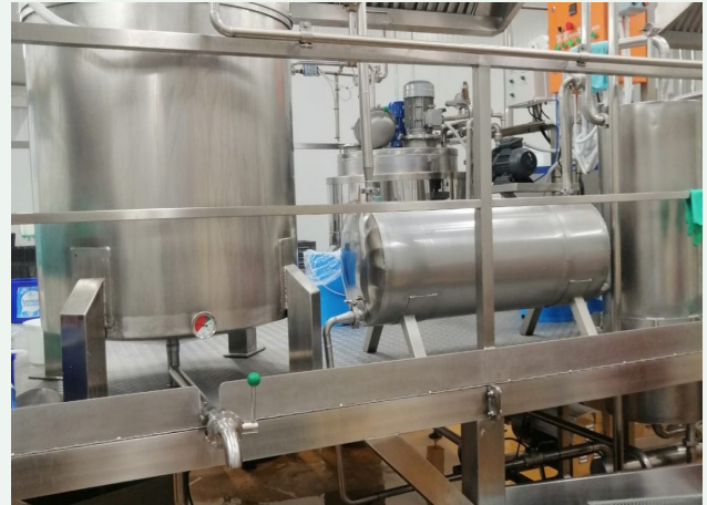
Process tanks and extraction canopy
