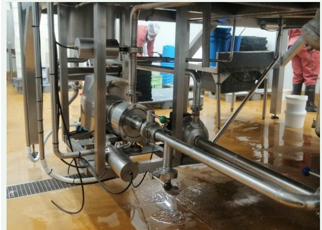
Process-line piping and pump assembly
