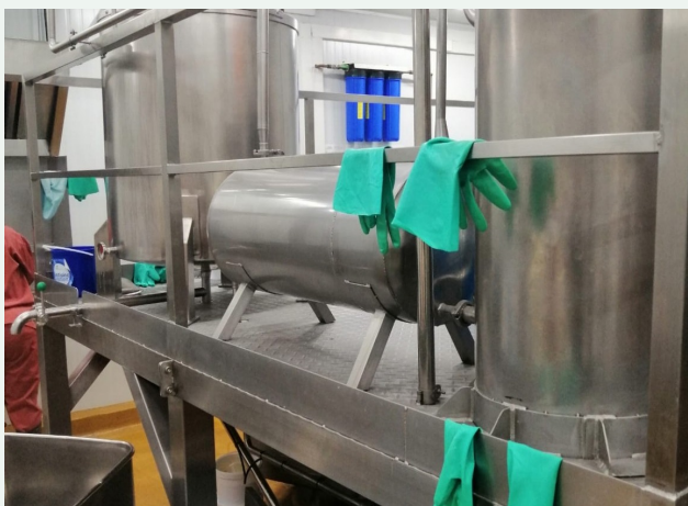
Stainless-steel tanks and support structure
